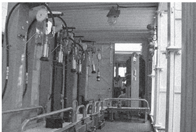
Figure A.6 LP Gas Supply Skids
